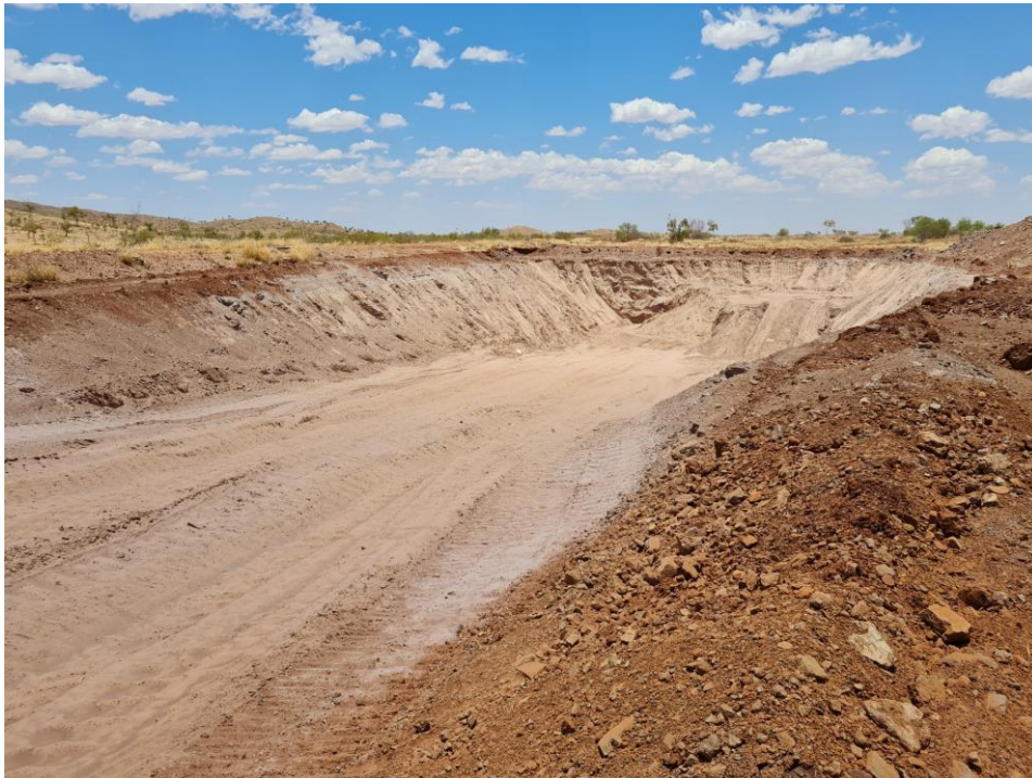
Figure 1 6,000t bulk metallurgical sample pit collected from the Tick Hill Tailings Dam Stockpile.
